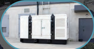
1,000 KW GENERATOR BRAND NEW 4,000 AMP SERVICE TO THE BUILDING
